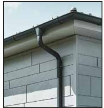
Rain Water Pipe
