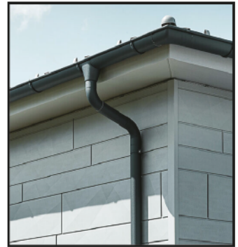
Rain Water Pipe
